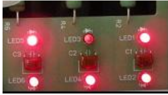
Fig. 2-13 Example of LEDs indication at open failure of arm on V phase of power module.
